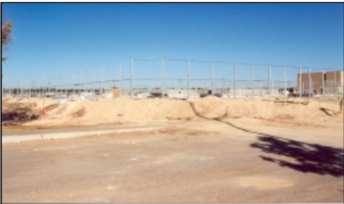
The NEW Tennis Center at Tech will be completed in time for the 2001 camp! Be the first to play on the state of the art facility.
